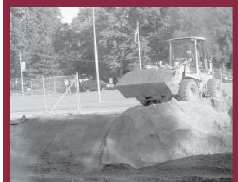
Crews begin the ground work for the construction of a new library addition at Saddlewood Elementary School. Several school projects got underway this summer.
