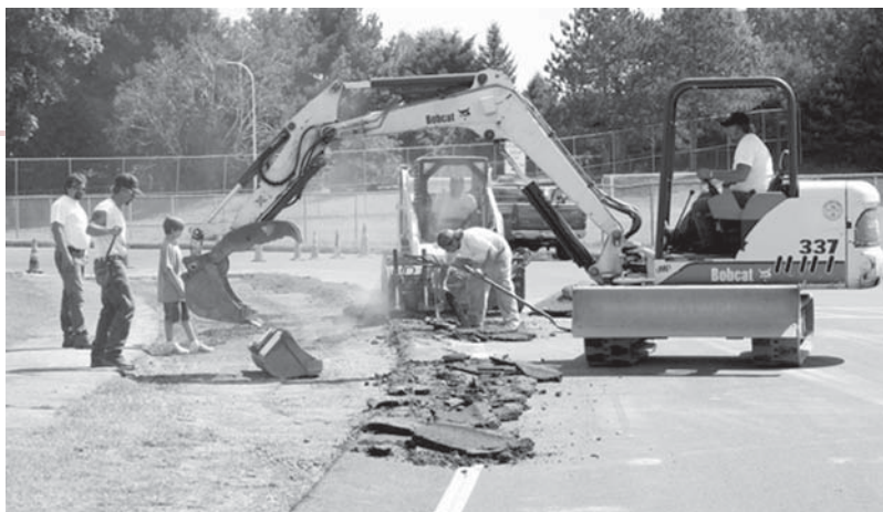
Crews install a new turn lane into the MUG off Raider Boulevard at Colonie Central High School.
