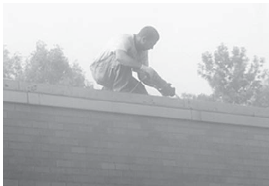
Construction crews tackle summer roof repairs/replacements at Colonie Central High School (top 2 photos) and Lisha Kill Middle School.
